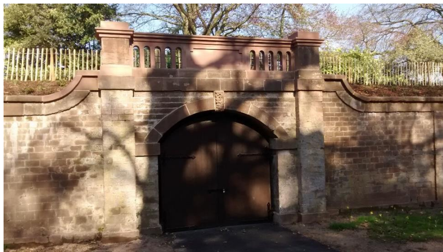
The restored Bier Store, with new balustrades above. Below right: the Non-conformist Chapel, awaiting restoration.
