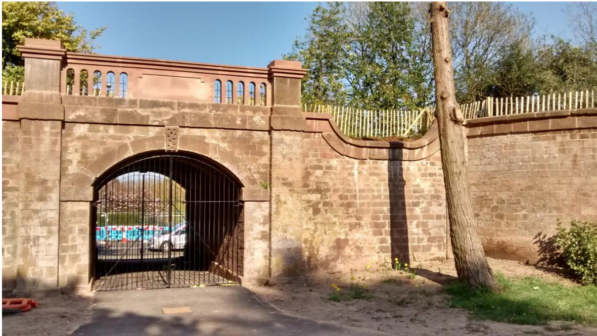
The restored carriageway gatehouse, viewed from inside the cemetery, looking out to London Road. Photos: John Marshall
