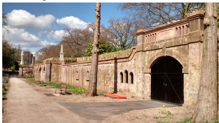
Viewed from inside the cemetery, the old carriageway entrance from London Road has been reopened and restored. The tunnel was bricked up in c1939 and the area used as an air raid shelter.
